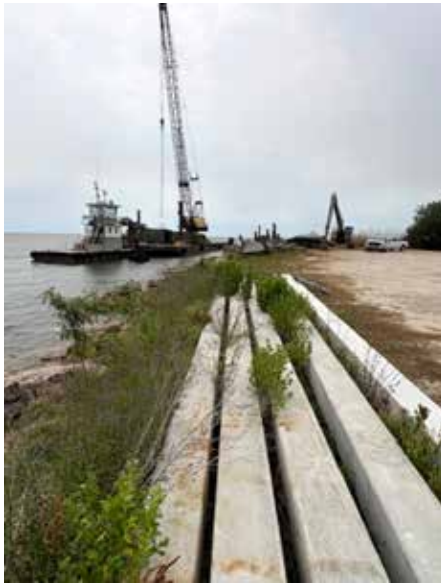
Work progresses on a million-dollar project using TDC funds to replace an important tourism pier in Apalachicola.
